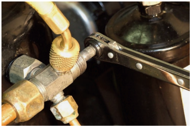
Figure 25-12 Square stem service valve and valve wrench
