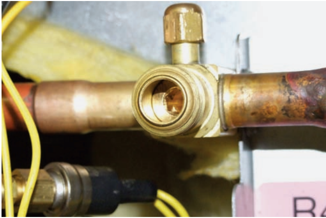
Figure 25-18 The condensing unit is shipped with the valve closed to hold in the system refrigerant
